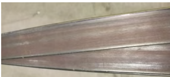
Figure 72: Small hairs of TPU sticking from rope surface Possible cause: manufacturing or installation.
