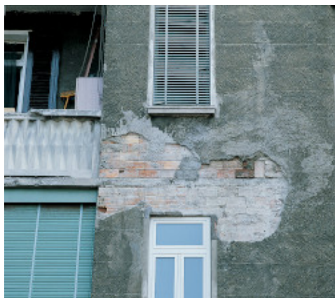
Degraded building façade in need of repair
